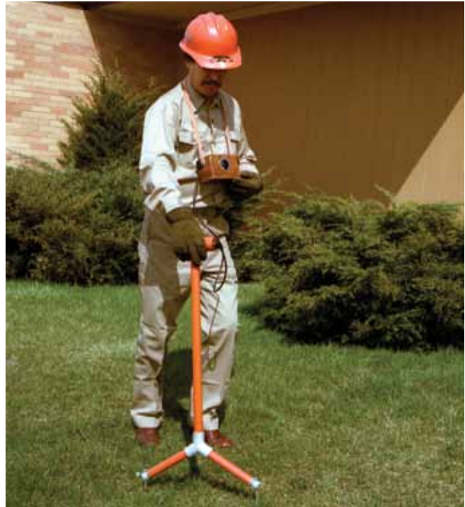
Locating the fault.
